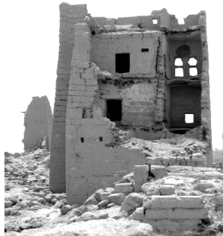
Photo 1 Adobe house destroyed by heavy rainfall [2]
