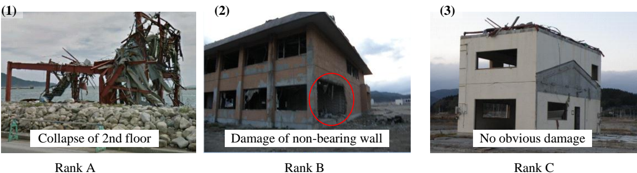
Fig. 5 Damage performance of buildings
