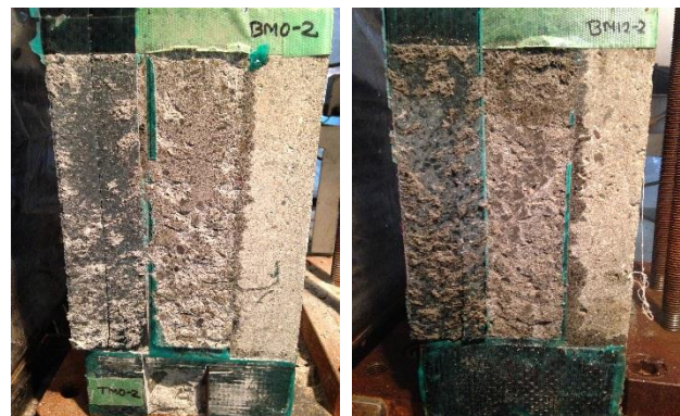
0 month 12 months Fig. 13 Partial concrete-resin interface failure before and after the exposure (Specimen BM type)
