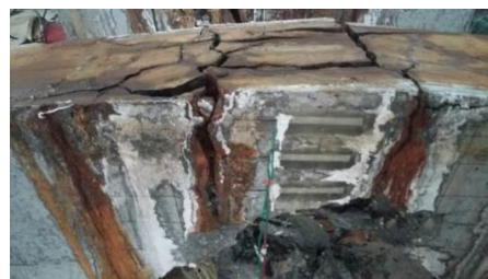
(c) Specimen of corrosion with cracks (F3)
