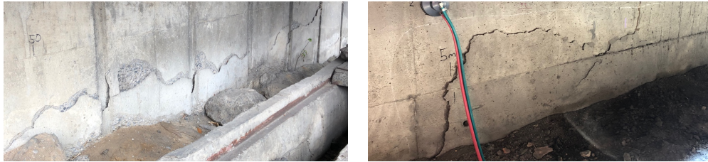
Fig. 1 Localized damage at two test locations (Left: W1-3, Right: W2-1)
