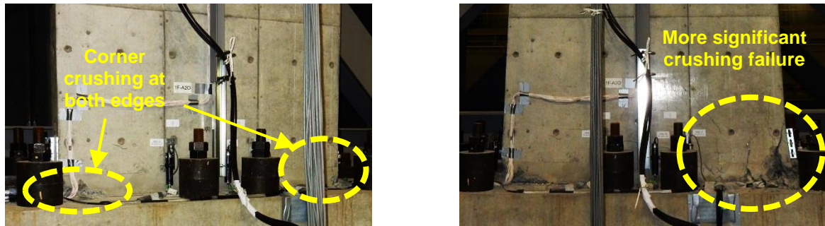
(a) After 1.5-scaled (first run) (b) After 1.6-scaled Fig.8 Progression of damage in 1F-A2 column base (insignificant damage observed after 1.0 scaled input and thus photo not included; significant damage indicated)
