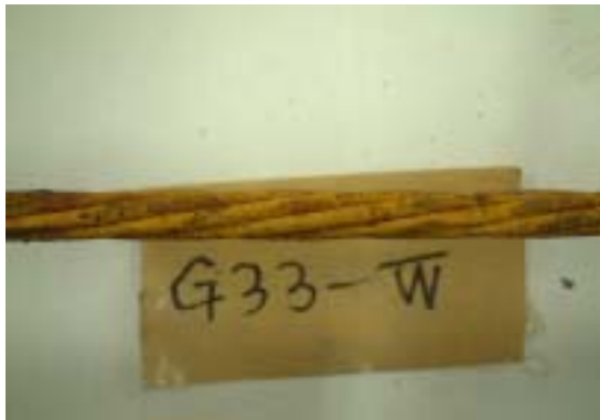
Fig.3 Corrosion of prestressing steel (Beam B8)
