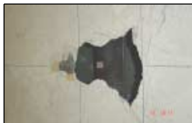
Fig. 4(d). Top view of punching shear failure, Control specimen-A1
