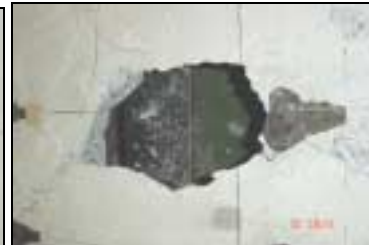
Fig. 4(e). Punching shear failure, Control specimen-B5
