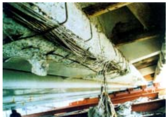
Fig.1 Deterioration of prestressing tendons [2]
