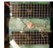
Photo 2 Cracks on specimen (Test series 2, without joint)
