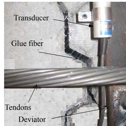
Fig. 13 Glue fiber at joint opening in SJ10-06
