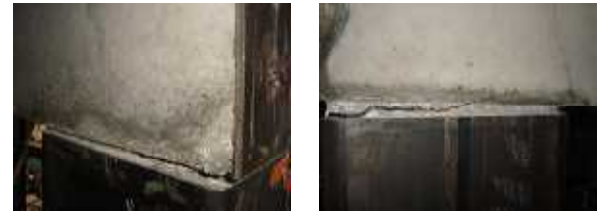
Photo.1 Fractures of columns
