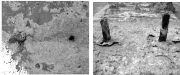
Fig.9 Anchor rupture and pullout of fiber anchors
