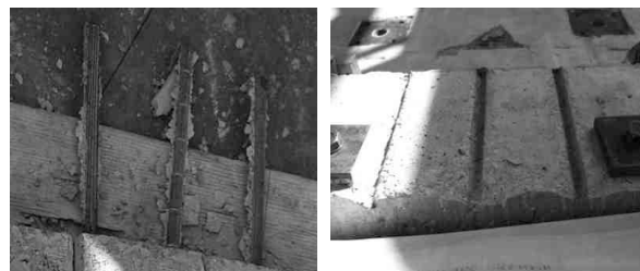
Fig.12 Anchor pullout of NSM anchors
