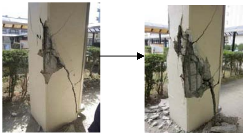
Fig.3 After 11 th of March earthquake
