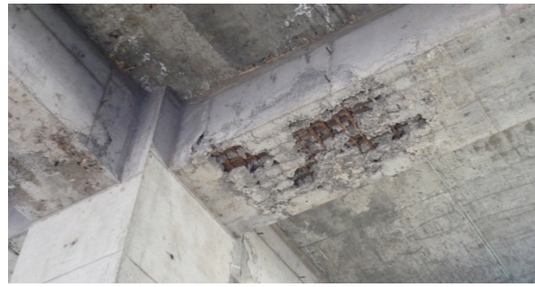
Photo 4 Example of low-quality surface concrete conditions in a large building under construction
