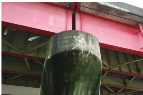
Fig.1 Bridge pier repaired with Na 2 SiO 3 compound and subsequently re-damaged by ASR in Toyama Prefecture
