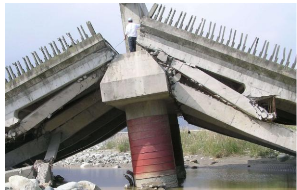
Fig. 4 Damage of P3 (view from downstream)
