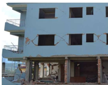
Fig. 1 Damage of Building with Masonry infill in 2015 Nepal Earthquake
