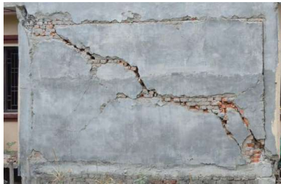
(c) Severely damaged RC frame with Masonry infill
