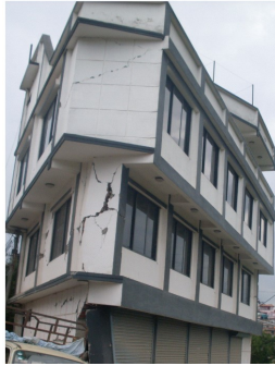
(a) Severely damage Irregular building
