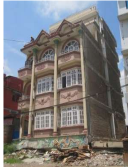
(b) Collapse due to soft story effect
