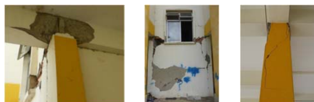
(a) Column (b) Infill wall (c) Column Fig. 2 Actual damage observed at the earthquake
